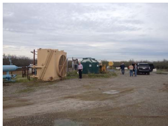
Figure 3: SGC Sacramento Gas Production Facility
