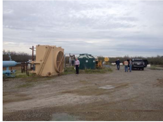
Fig 3: SGC Sacramento Gas Production Facility
