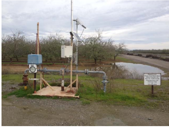
Fig 2: SGC Sacramento Basin Meter Station
